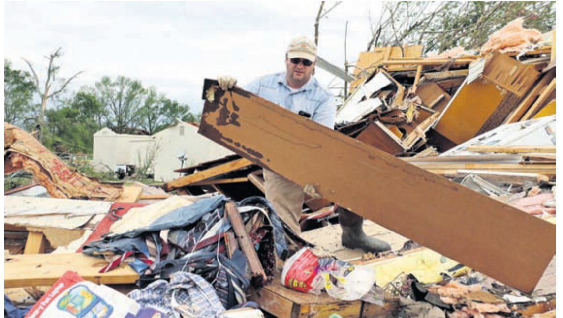
Roman Brown moves part of a wall out of his way as he looks for a friend's medicine in their destroyed home along Seely Drive outside of Hamilton, Miss. after a storm moved through the area on Sunday, April 14, 2019.
